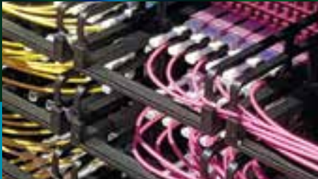
HIGH-DENSITY DATA CENTRE SOLUTION (HD-DCS)
