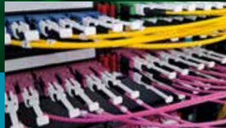
MEDIUM-DENSITY DATA CENTRE SOLUTION (MD-DCS)
